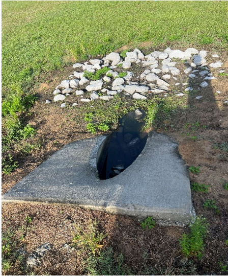
Erosion Around M.E.S. (typ.)
