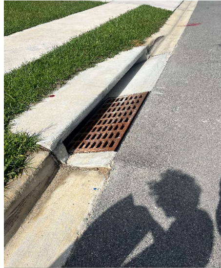
Misaligned Concrete & Asphalt Along Inlet
