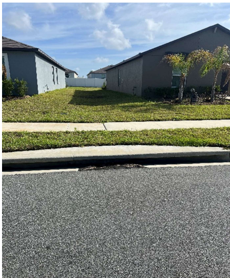
Stormwater Inlet Blockage (typ.)
