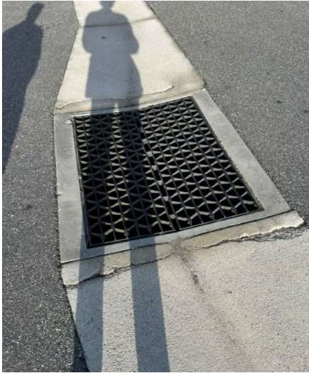
Cracked Concrete Along V-Inlet
