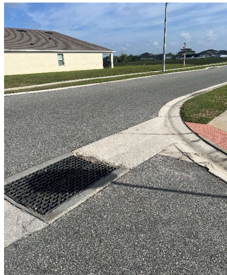
Cracked V-Inlet and Curbing Concrete
