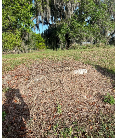
Overgrown Outfall Structure (typ.)
