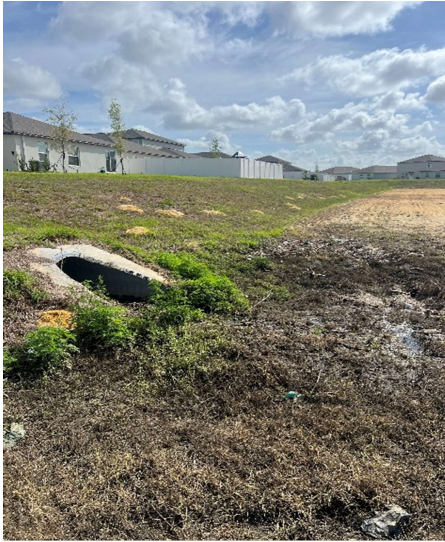
Damaged M.E.S. & Pond Debris
